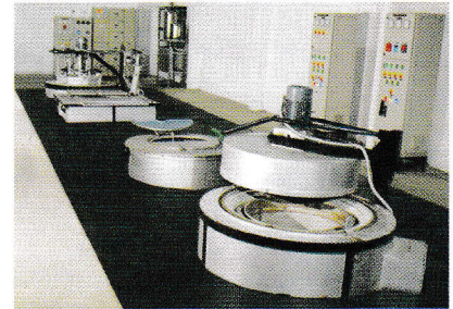
Heat treatment plant
